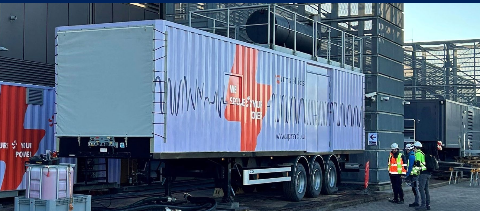
(Photo 7 - Mobile UPS System Luminus Solutions)
