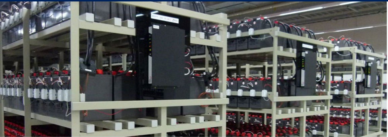
(Photo 2 - battery storage)
